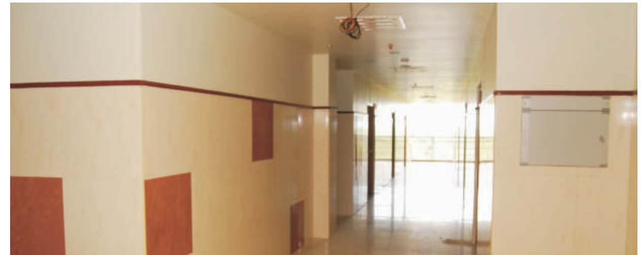
CERAMIC AND VITRIFIED TILES ARE WET CLAPPED ON TO THE FIBRE CEMENT BOARD USING TILE ADHESIVE
